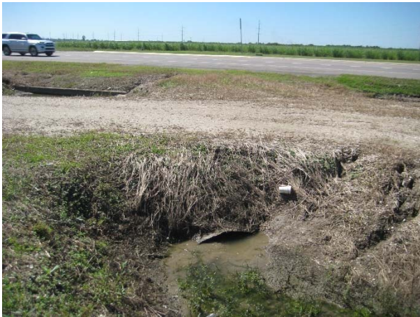
Picture 17C: Looking south at culvert 105-2 (Buried). North Canal Blvd. in background. (Reference E-4.1)
