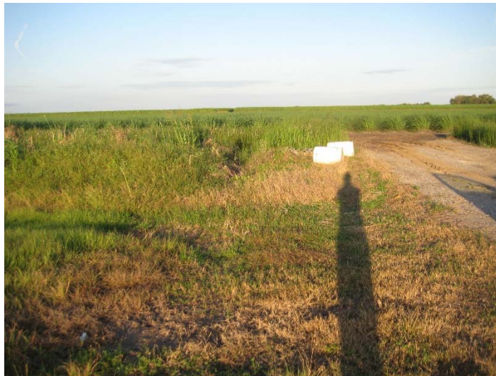
Picture 3I: Remains of emergency weir cut by the city of Thibodaux during past heavy rain event to drain the St. Patrick Street roadside ditch. (Reference E-2.2)
