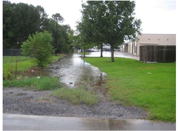
Picture 5F: Sub-lateral 102B looking north from station 312+70 (James Riviere St.) (9/26/2018 Rain Event) (Reference E-2.4)
