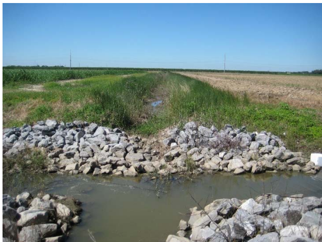
Picture 13A: Sub-lateral 103E looking west from North Canal Blvd. at station 608+00. (Reference E-3.5)
