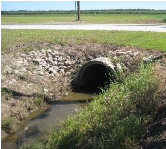
Picture 13E: Looking east at culvert 103E-2. Swanson Drive in Background. (Reference E-3.5)
