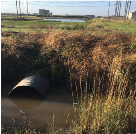
Picture 12C: Concrete outfall structure 1 discharge culvert into Sub-lateral 103D (Reference E-3.4)
