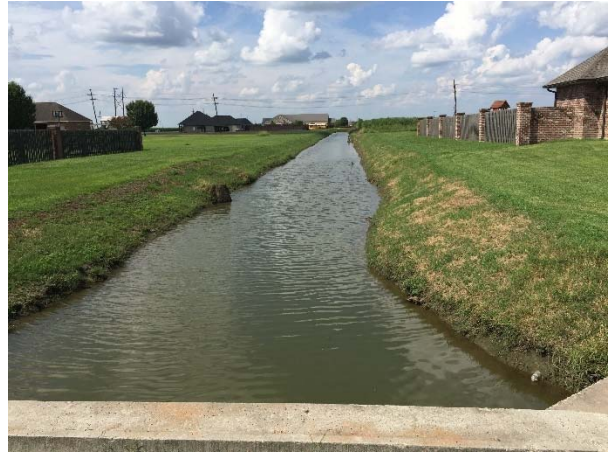
Picture 10F: Sub-lateral 103B looking north from station 328+00 on Concrete Bridge Structure 2. (Reference E-3.4)
