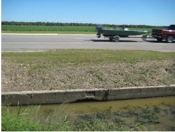
Picture 15A: Looking east at culvert 104A-1. North Canal Blvd. in background. (Reference E-4.1)
