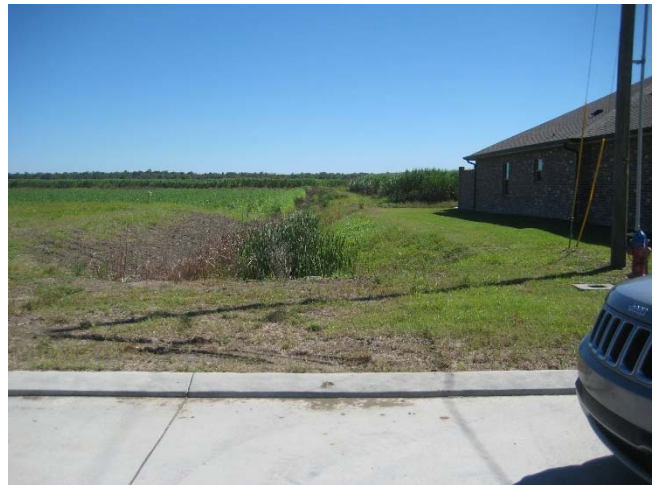
Picture 13F: Sub-lateral 103E looking east from Swanson Drive at station 618+25. (Reference E-3.5)
