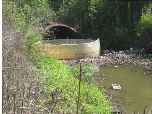
Picture 1G: Looking north at culvert 101-8 (obstructed) at station 110+00 (8/30/2018) (Reference E-1.3)
