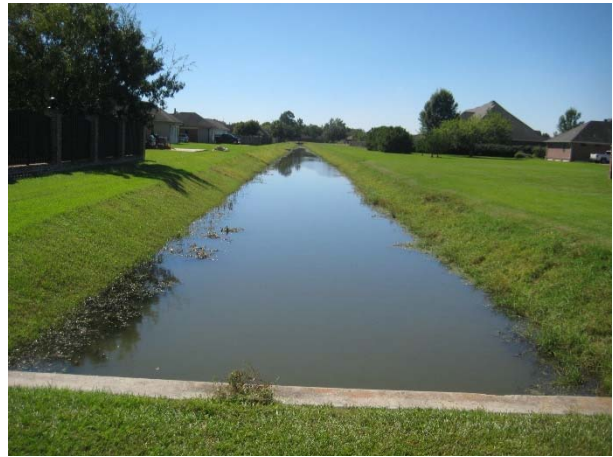
Picture 10B: Sub-lateral 103B looking south from station 314+50 @ Concrete Bridge Structure 1 (Reference E-3.4)
