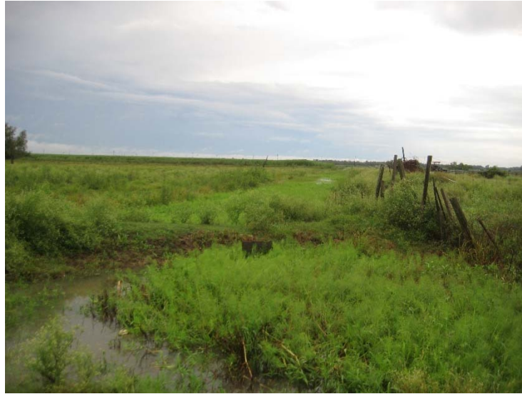
Picture 15E: Sub-lateral 104A looking west from station 242+00. Blocked culvert shown. Rienzi Canal in foreground. (Reference E-4.2)
