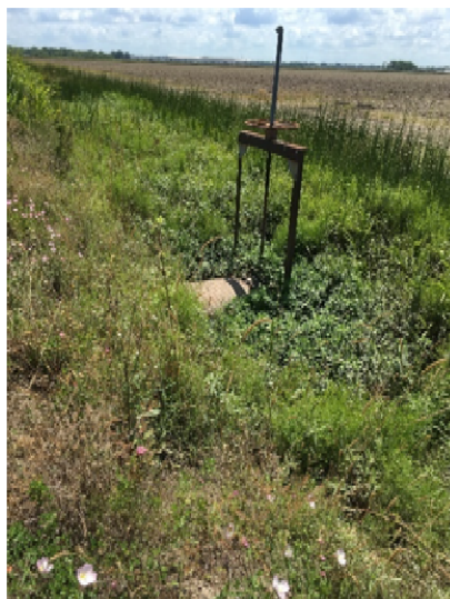
Picture 12: Manual sluice gate 2 at the upstream end of lateral 103D, discharging into Lateral 102. (Reference E-3.4)
