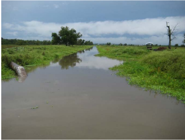
Picture 8G: Lateral 103 looking south from station 128+00. Private pump discharge pipe shown. (Reference E-3.3)
