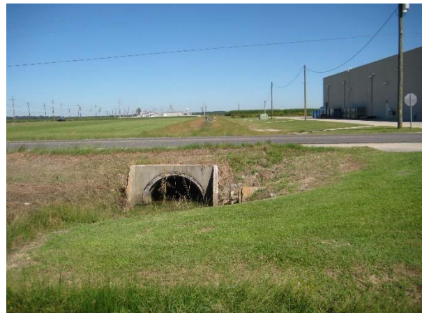
Picture 11B: looking north at culvert 103C-1 under Glenwild Drive (Reference E-3.4)
