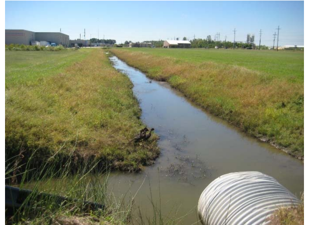
Picture 11D: Sub-lateral 103C looking south from station 415+00. Culvert 103C-2 in foreground. (Reference E-3.4)
