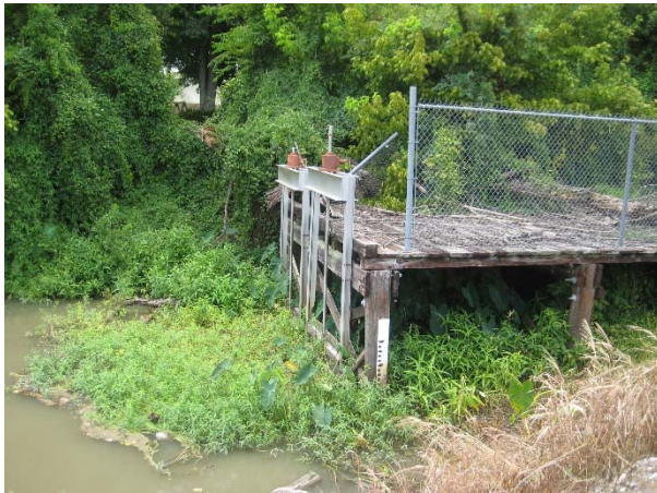
Picture 8A: Manual Sluice gate #1 within Lateral 103 at Bayou Lafourche (Reference E-3.1)
