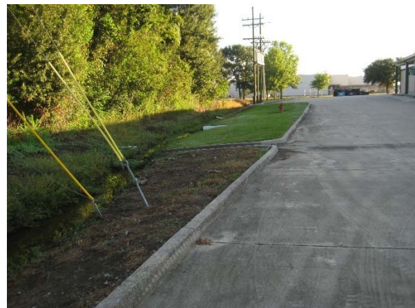
Picture 5H: Sub-lateral 102B looking north from station 315+00 (Limited Room for Widening) (Reference E-2.4)
