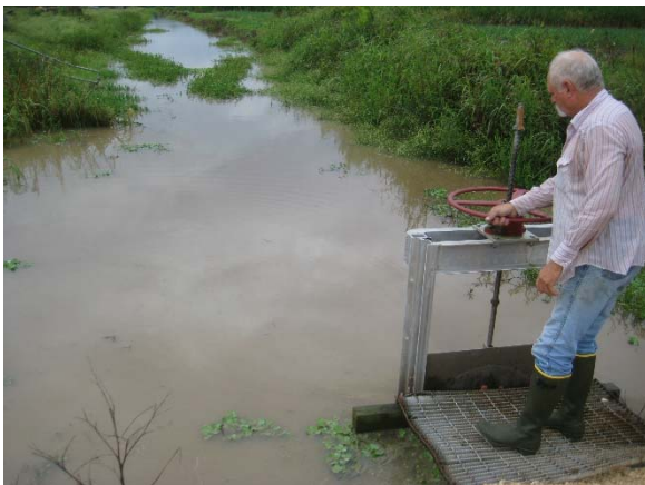
Picture 14F: Looking east at manual sluice gate 3 on east end of culvert 104+6. (Reference E-4.1)
