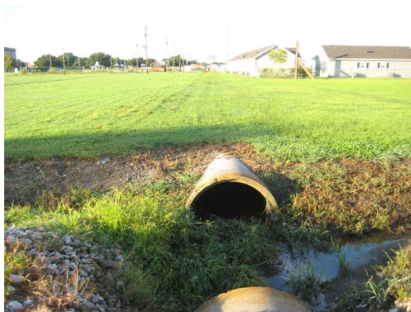
Picture 5C: Sub-lateral 102B looking south from station 312+50 (James Riviere St.) at culvert 102B-2 (Reference E-2.4)
